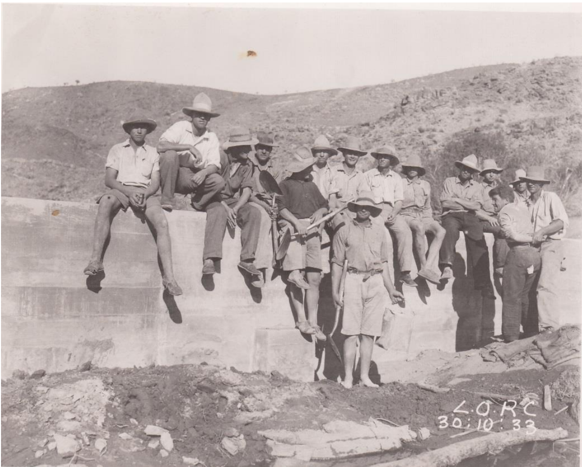
Indigent white workers at the Buchberg construction site (Source: K. Visser, Private Collection)
